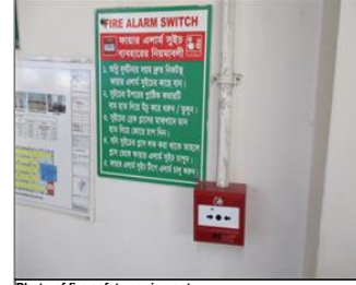
Photo of fire safety equipment Fire safety to confirm sustenance- Fire alarm.JPG
