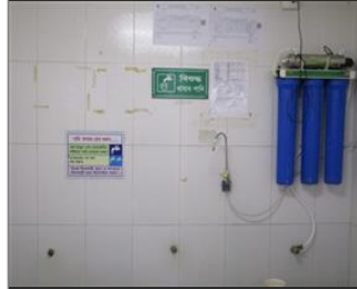
Photo of the sanitary facilities Drinking water.JPG
