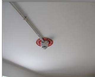
Photo of fire safety equipment Fire safety to confirm sustenance- Smoke detector.JPG
