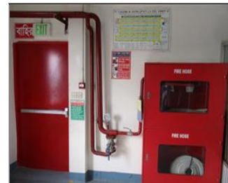
Photo of fire safety equipment Fire safety to confirm sustenance-Fire equipment.JPG
